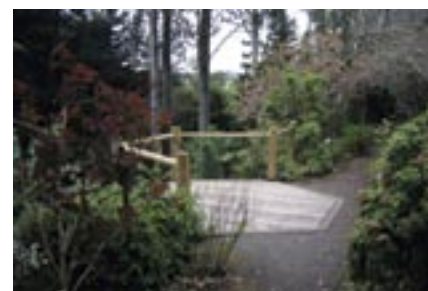
Fig. 7 At Ayrilies, attention is drawn to the best viewpoint and most dramatic topography by screening the less interesting features and building this simple lookout – out over a bank to add drama.
