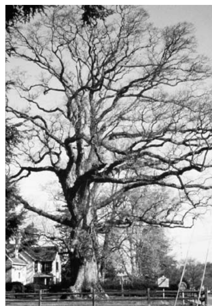
Fig. 7 Tall heritage tree showing the potential risk to an adjacent building.
