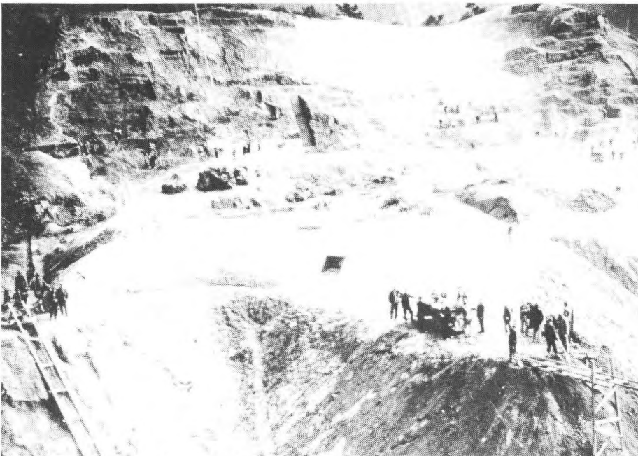
Fig. 5. Central Western Town Belt 1932. Anderson Park extension under construction. Providing social welfare has played a large part in shaping the Town Belt. Land has been taken for hospitals, or hills have been flattened in the process of providing outdoor relief. Today the Rose Garden and Begonia House occupy this site. Photograph: Evening Post Collection, Alexander Turnbull Library.
