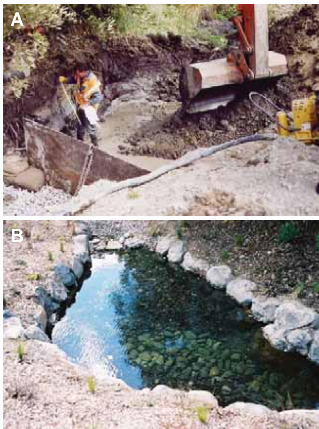
Fig. 12 Excavation of deep pools provides aquatic refuge when flow stops and also act to trap sediment reducing extent of siltation downstream. A , during construction; B , completed pools.
