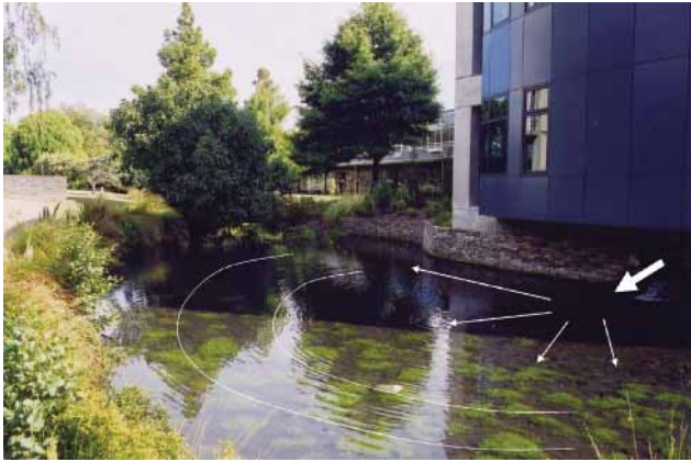
Fig. 4 Previous flow pattern showing how air-conditioning water discharged from a School of Engineering building impeded flow by pushing water upstream. Photo taken looking upstream. Arrows indicate water flow patterns.
