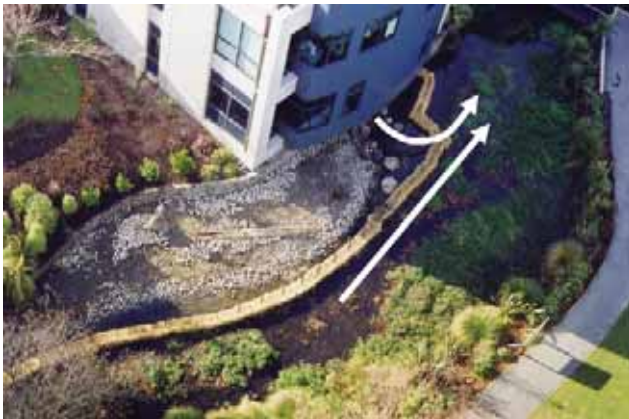
Fig. 6 Gravel bar constructed to redirect air-conditioning discharge flows and to narrow the stream. Hay bales were used as sediment control during construction. Arrows indicate water flow patterns.
