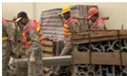
Fig. 16 The old fashioned method of transferring heavy granite stones by hand for the bridge might not appeal to New Zealand tradesmen but was a quick and efficient means of moving heavy objects in a tight space with no room for machinery.
