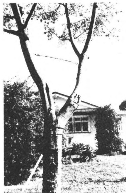
Fig. 4. The home made cable bracing in this Melia azederach will not help the trunk knit together.
